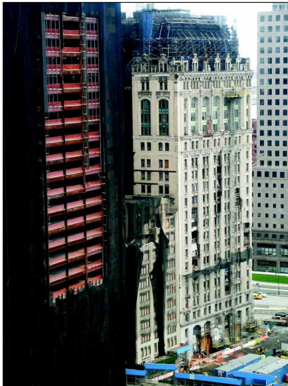
DUST DEVIL — A chain-mail like cloth drapes over the Deutsche Bank building at 130 Liberty Street (left) in Lower Manhattan last year. A 15 story gash was created when steel girders from World Trade Center Tower 2 fell on the Deutsche Bank's northern face on Sept. 11, 2001. Tons of hazardous debris from the collapsed towers shot into the building which is still there today.
